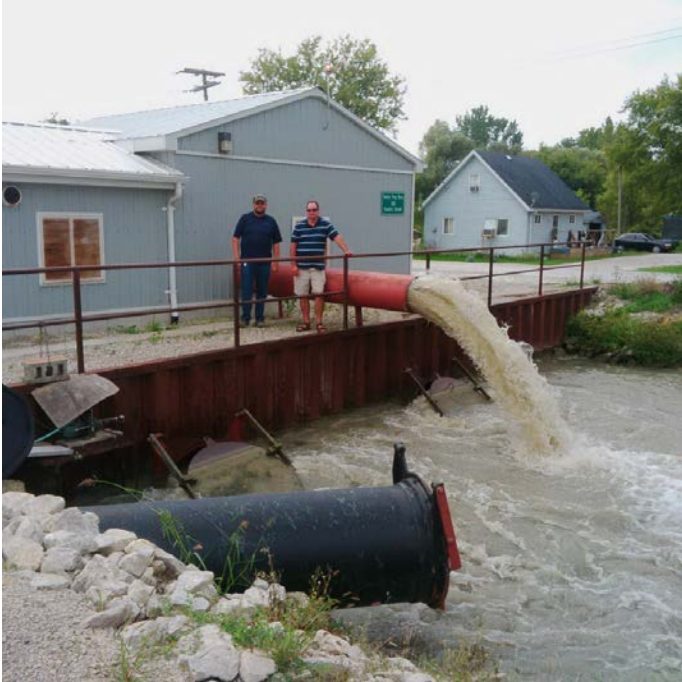
Municipal drain pumping station in Chatham-Kent Credit: Nicola Crawhall, Cities Initiative
