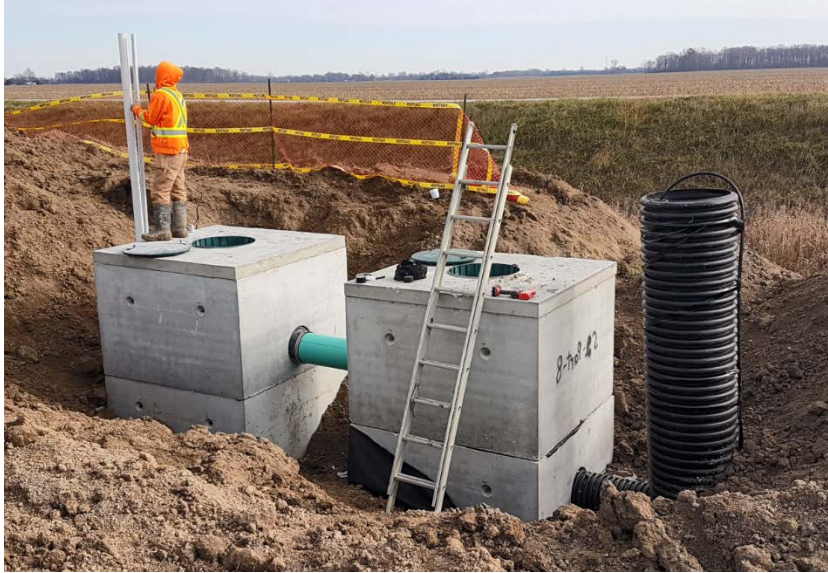
Installation of a surface water filtration box system in Chatham-Kent Credit: Kevin McKague, OMAFRA
